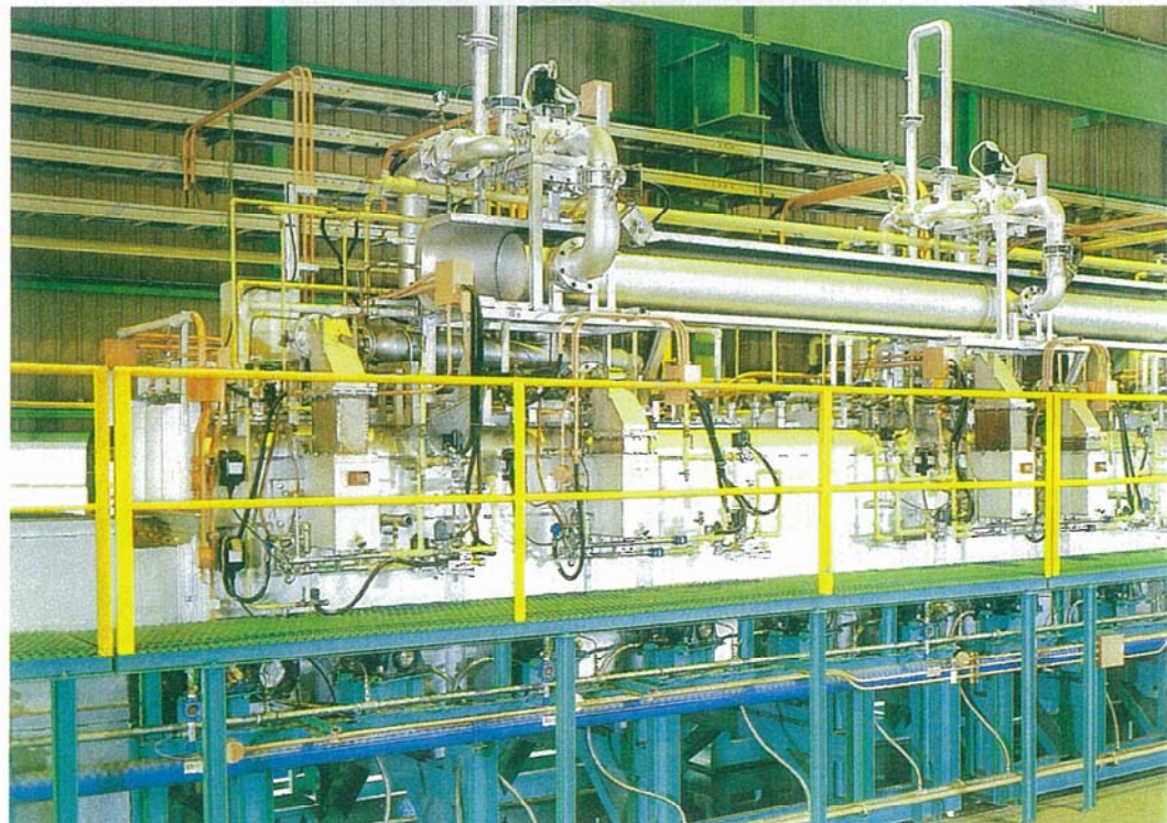
Roller Hearth Type Heat Treatment Furnace 5 t/h Daiichi Netushori Steel Co., Ltd. Muroran, Hokkaido
